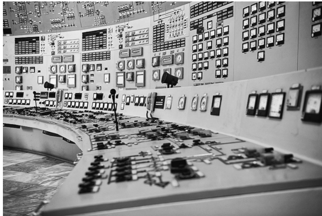
Figure 3: A set of electro-mechanical panels in a nuclear power plant control room (© 2009 Yovko Lambrev. Creative Commons)
